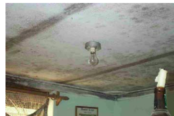
Mould grown on a ceiling
